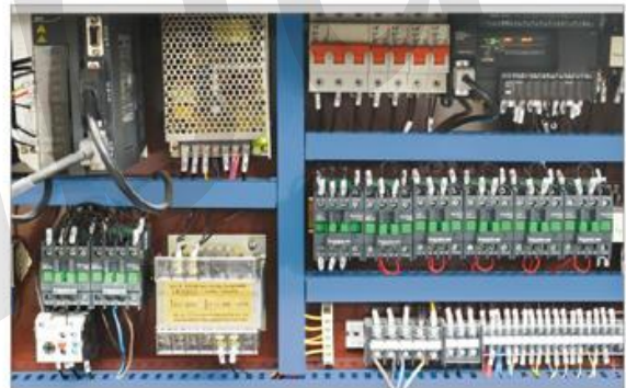
电器箱 Electric Cabinet
